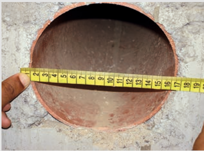
KG pipe misused as wall sleeve
