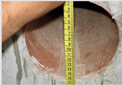
KG pipe as wall sleeve
